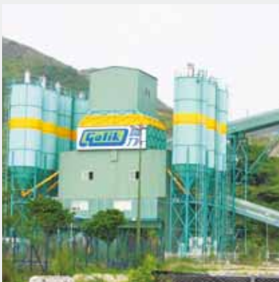
Ready Mixed Concrete Plant in Siu Ho Wan, Lantau Island, Hong Kong
